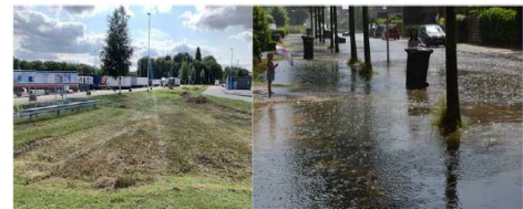
Figure 9.44 Diminished functioning of SUDS. Left: Maintenance with heavy equipment leads to compaction of the soil (Source: https://www.climatecan.org/projects/6915/detail ). Right: Insufficient hydraulic capacity of a swale and road flooded with stormwater (Source: https://www.climatecan.org/projects/210/detail ).
