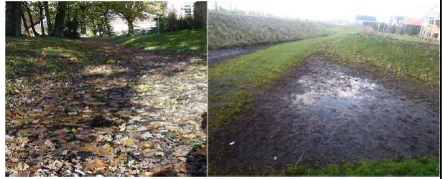
Figure 9.40 Left: Dutch Swale in Enschede (Ruwenbos) littered with leaves. Right: Clogged swale at Haarzicht Utrecht. Source: https://www.climatecan.org/projects/7921/detail .
