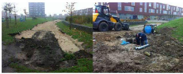
Figure 9.41 From left to right: Removing of top layer swale (construction 2000) due to clogged layer in 2012, Nijmegen, replacement of drainage pipes and removing top layer swale (construction 2007) due to clogged layer in 2012, Nijmegen. Source: https://www.climatecan.org/projects/4364/detail .
